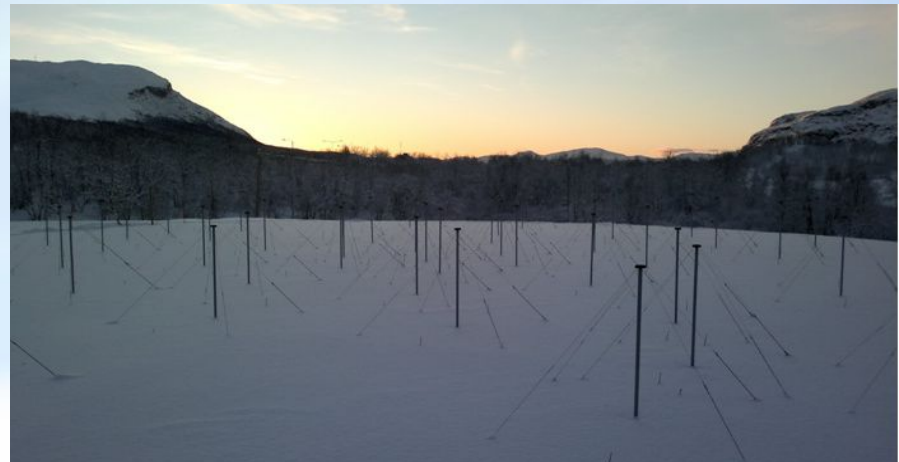
Low-Band Antenna (LBA) array 34 m diameter 48 aerials 10-90 MHz
